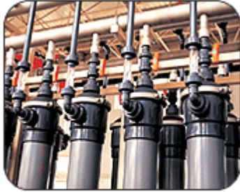
Continuous membrane filtration system 连续膜过滤系统
